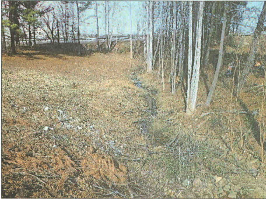
The South Carolina Department of Transportation cleared about half of the area. [NEWT HARDIE]
